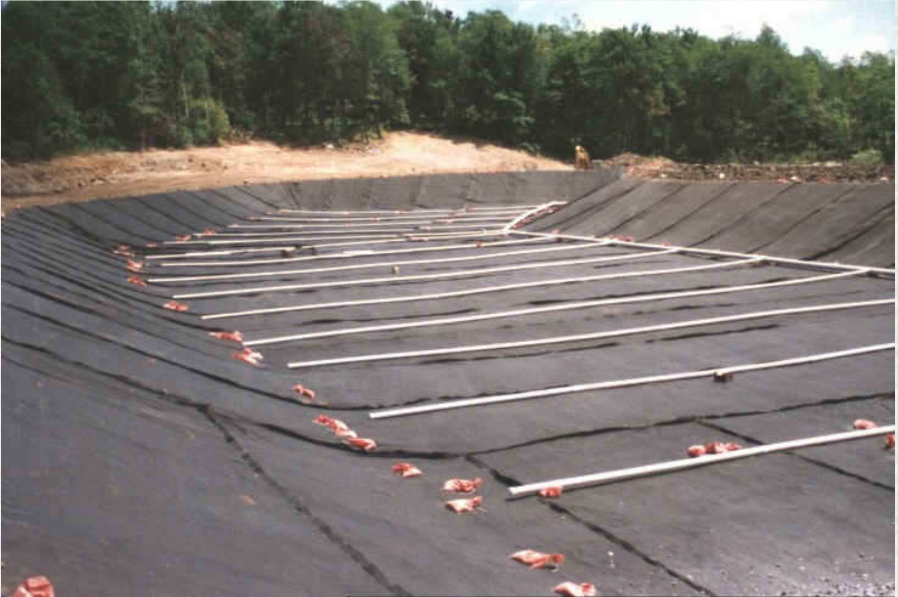
PIPING SYSTEM IN TREATMENT CELL
